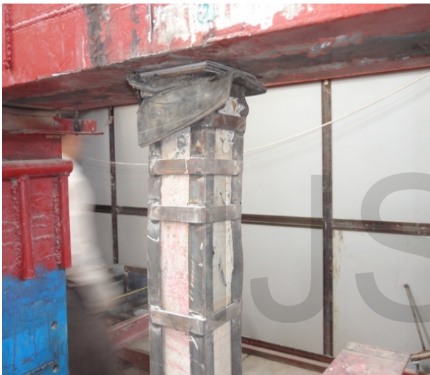
Figure (13) The failure pattern of strengthened column
