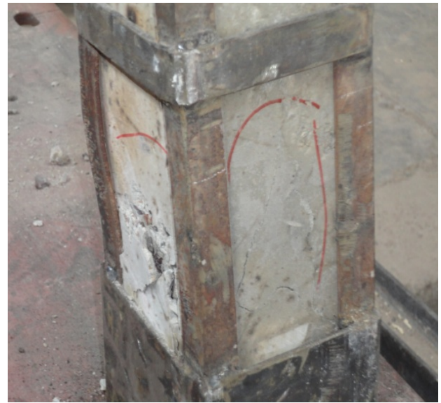
Figure (14) The failure pattern of strengthened column
